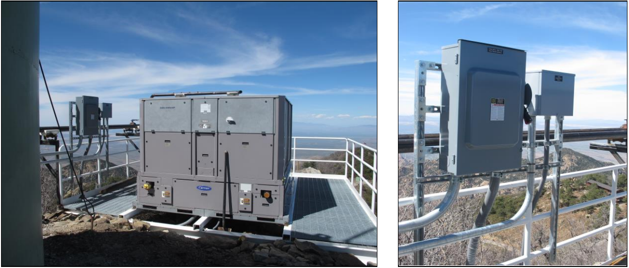
Figure 2. Shown are power and network control connections completed for the second Carrier chiller (left), also known as “CH2” and “Carrier-on-the-Rock.” New junction boxes and plumbing (right), mounted to the left of the CH2 unit, were installed during this reporting period. The view is to the southeast from behind the support building at the summit. Work will continue on integrating this Carrier CH2 chiller into the HVAC and M1 ventilation system. The HVAC system is being configured so that cooling can be quickly changed between this second chiller (CH2) and the existing chiller (CH1). These two chillers will eventually be integrated into an upgraded HVAC system, using the BACnet network protocol.
