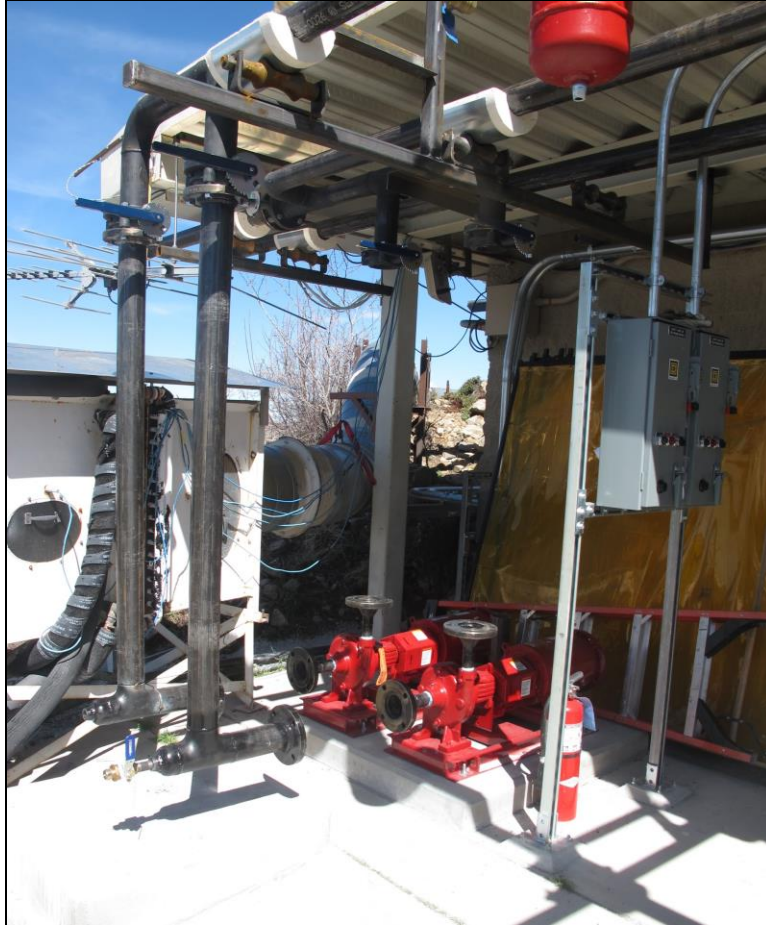
Figure 3. New red glycol pumps were installed next to the shop heat exchanger, shown on the left. The two new pumps will soon be connected to the newly upgraded HVAC system. These two 10-horsepower Bell & Gossett Series E-1510 pumps will greatly increase the glycol circulation capacity of the HVAC system. Additional new plumbing and electrical work is also shown in the photo. Work on the HVAC system will continue into the summer.
