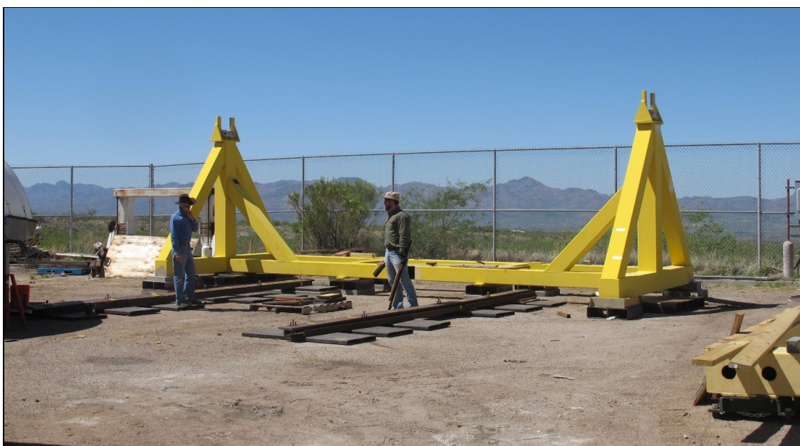
Figure 1. This image taken during the grouting process shows the tilt frame and bell jar cart tracks in position.
