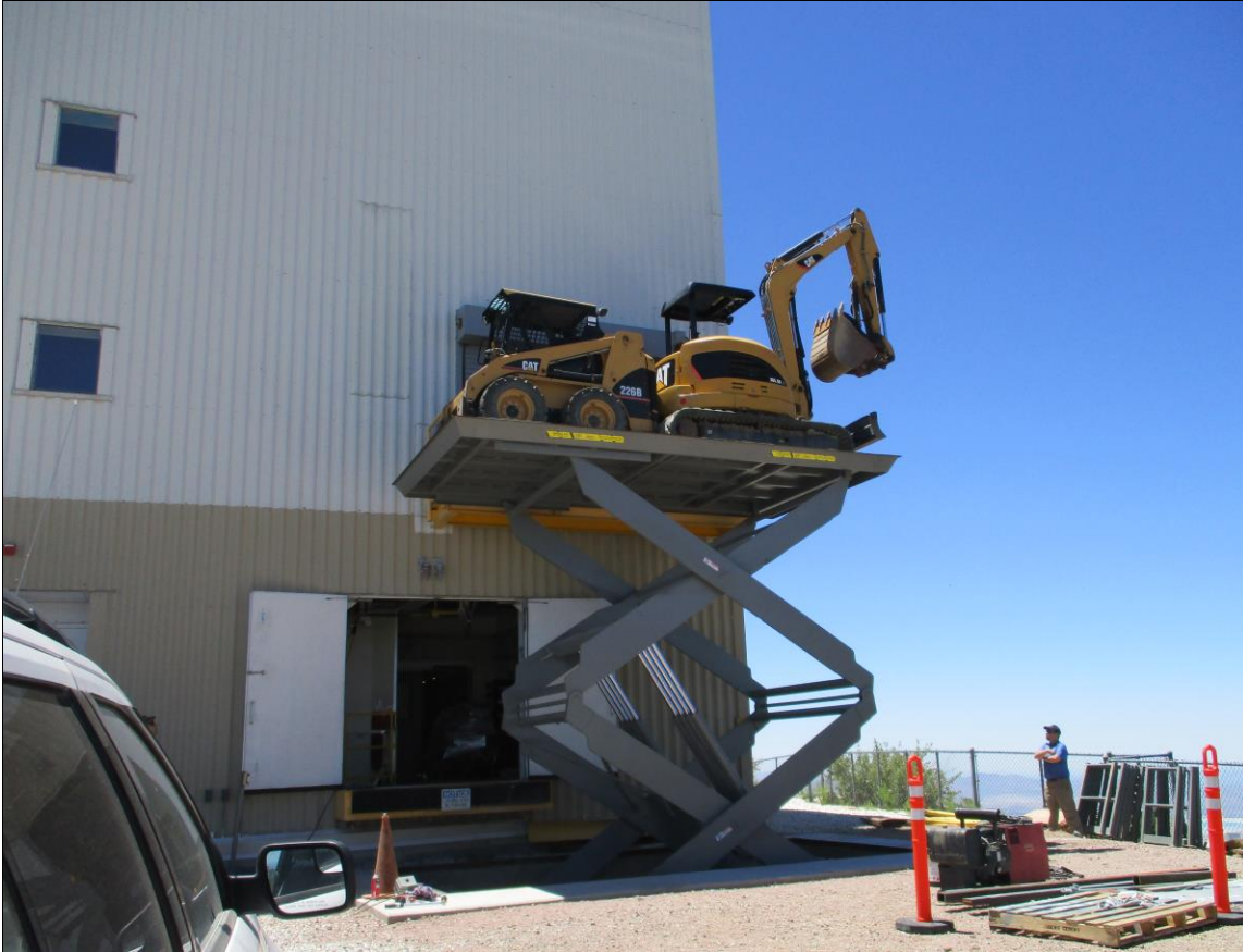
Figure 8. Load testing of the outside equipment lift. A safety monitor is in position to the right of the lift. Since the safety railings for the in-ground pit had not yet been installed, a safety monitor was used to ensure that personnel did not come near the pit while the lift was up. Limit switches and the railing system around the in-ground pit are expected to be installed in the fall. After thorough review of the job hazard analysis, a limited number of MMTO staff received approval to operate the lift.
