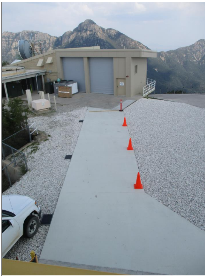
Figure 9. Completed concrete pathway for moving instruments between the telescope enclosure and the IRF.
